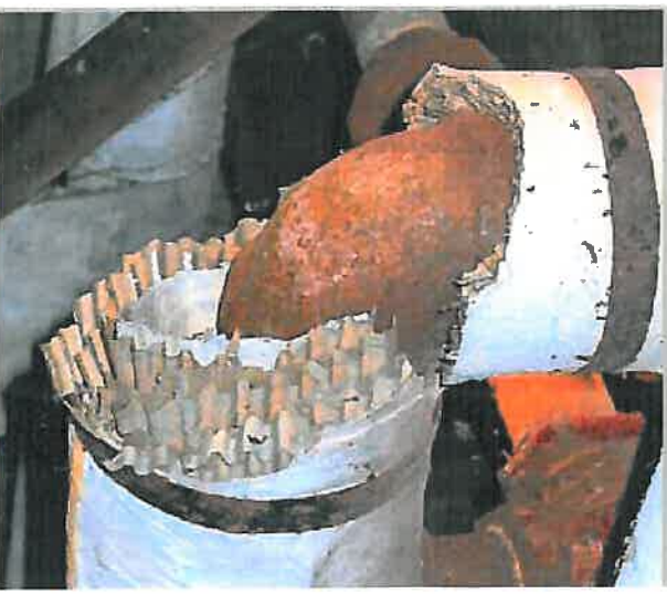
Damaged asbestos pipe insulation.
