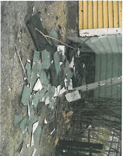
Improperly removed asbestos from home renovation project.
