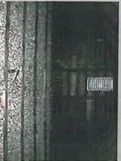
Vermiculite insulation found in an attic.
